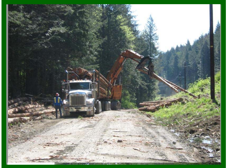
Transmission line right of way clearing for Southern Communities Grid Connection Project.
